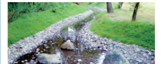
Example of recycling: revetment material (Photo: provided by Chuo Denki Kogyo Co., Ltd.)
