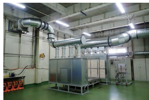
Reinforced pretreatment equipment (in the low-concentration PCB pretreatment building)
