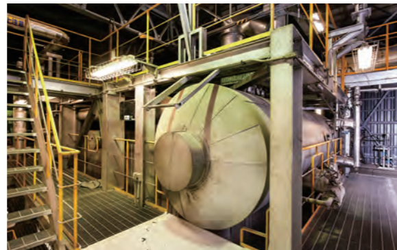
①Boiler This cools the combustion gas and supplies the generated steam to the on-site equipment and power generation equipment.
