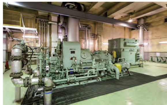
②Turbine Generator This generates power with the steam produced in the boiler. The generated power is used within the plant, and the surplus power is sold.
