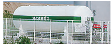
Carbon Dioxide Gas Injection Equipment (Photo provided by Togami Water Source, Yonago City)
